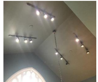
ZIGI mini-PAR lights installed as track lights
